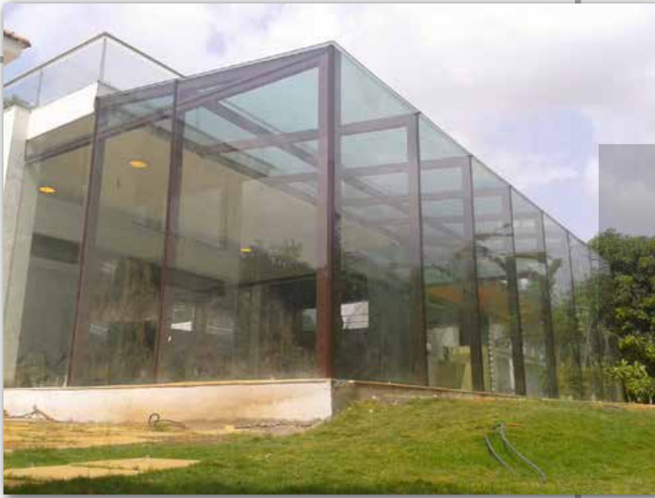
Facade Mild Steel Frame With Aluminium Composite Panel With Glass
