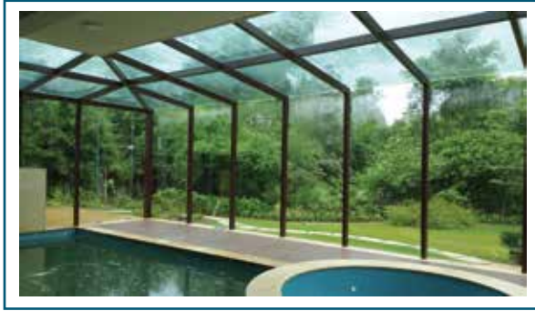
Facade Glazing - Dharampur
